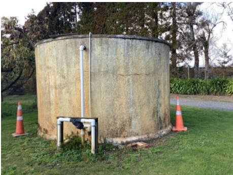
Water holding tank
